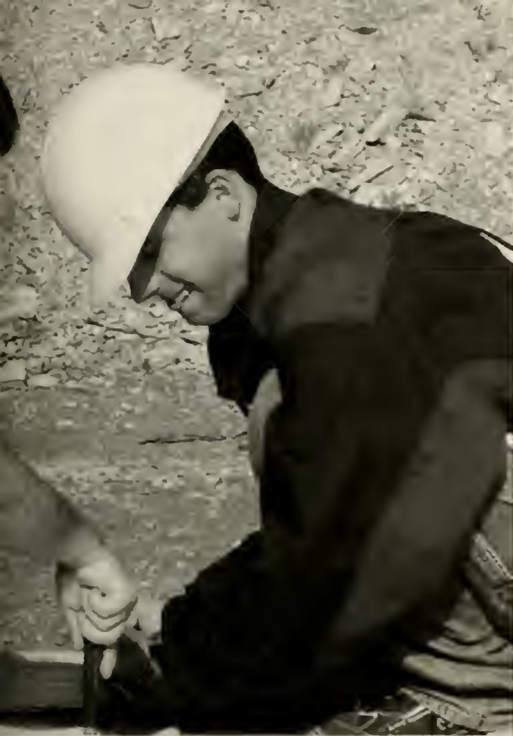
Setting the foundation, sophomore David Martin and junior Ryan Eades help on APOs Habitat for Humanity trip. The brothers traveled to West Virginia to build houses for the less fortunate. [ Photo courtesy of APO ]
